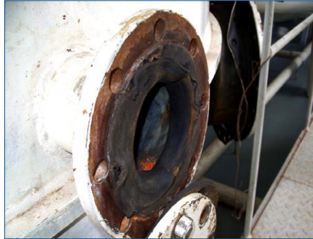
Corrosion damages on flange
